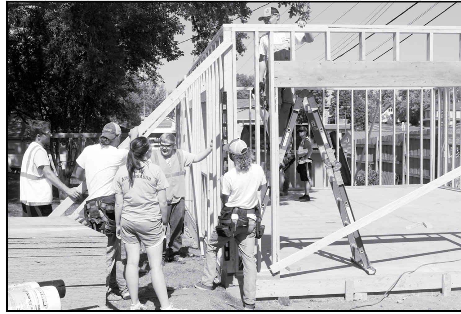
Wayne State College students involved in construction classes work on a garage as one of this semester's projects.
